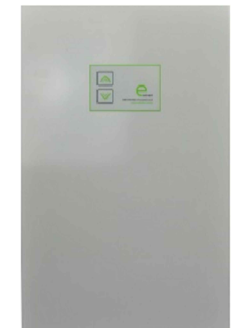
VENT 6 CONTROL PANEL
